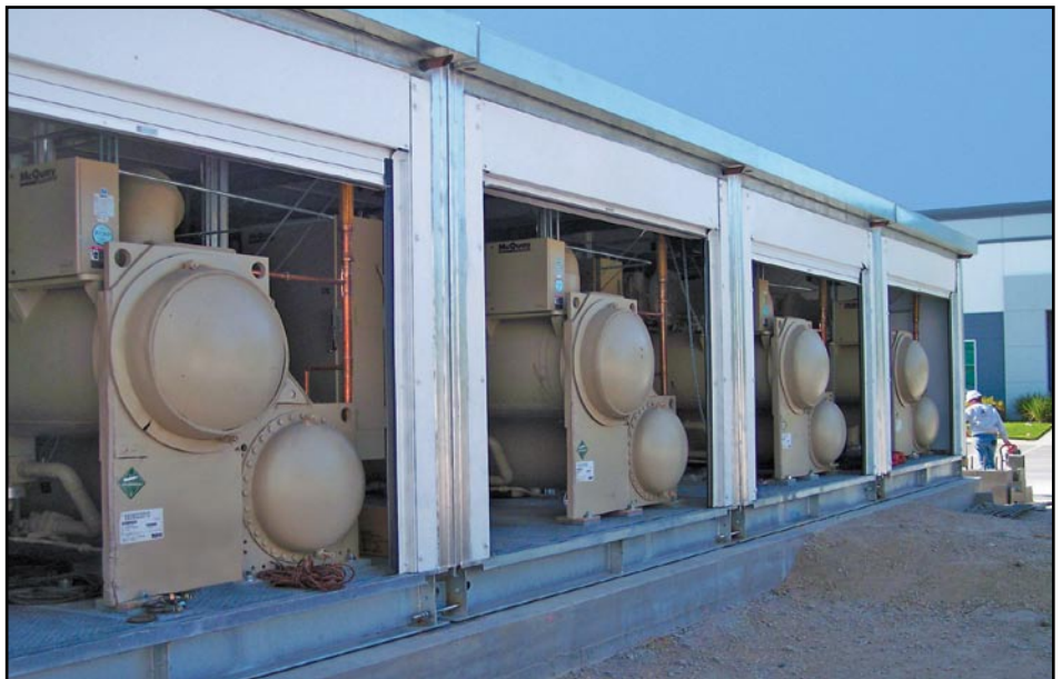
Four of the six McQuay Modular Central Plants that provide mission critical cooling for the Herakles Data Center.
