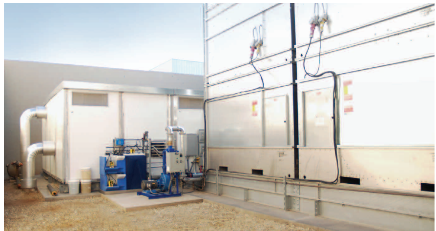
The water treatment pump and water filtration system on the Modular Central Plant are installed externally at the Arizona high school.
