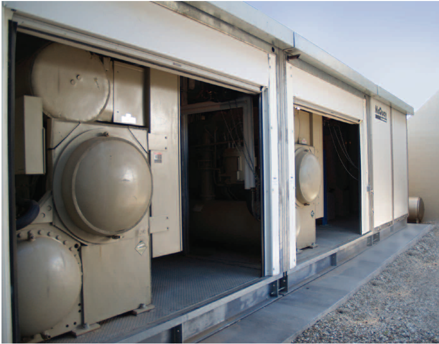
The Modular Central Plant at Chaparral High School features two energy efficient, 475-ton McQuay centrifugal chillers.
