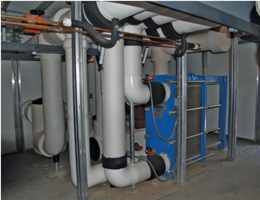
The Modular Central Plant at the school includes a plate-and-frame heat exchanger with secondary pumping.
