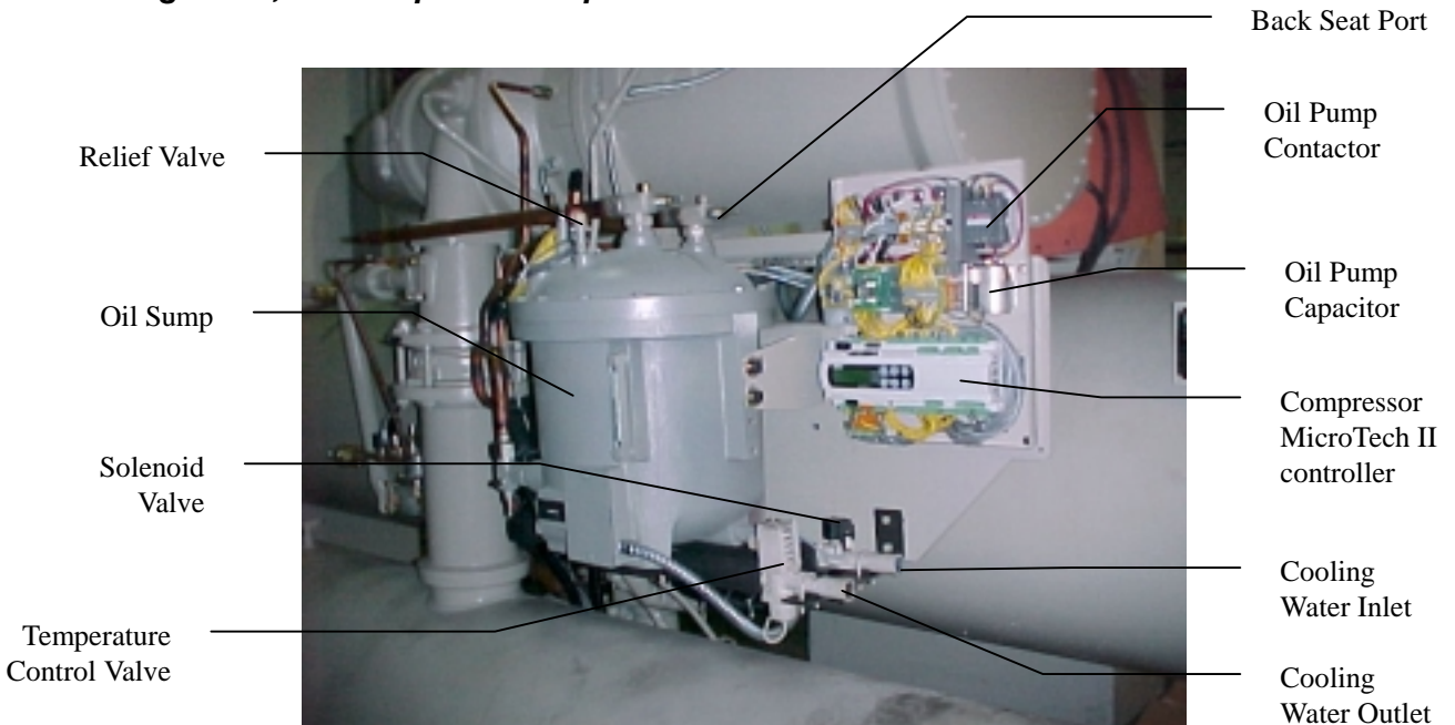
Figure 11, Oil Sump and Compressor Controller Panel
