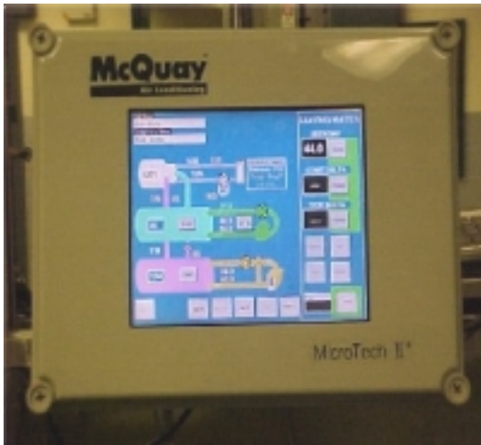
Figure 9, MicroTech II Control Panel
