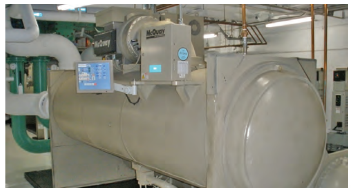
One of two 500-ton Magnitude Chillers installed at the Sarasota Bradenton International Airport
