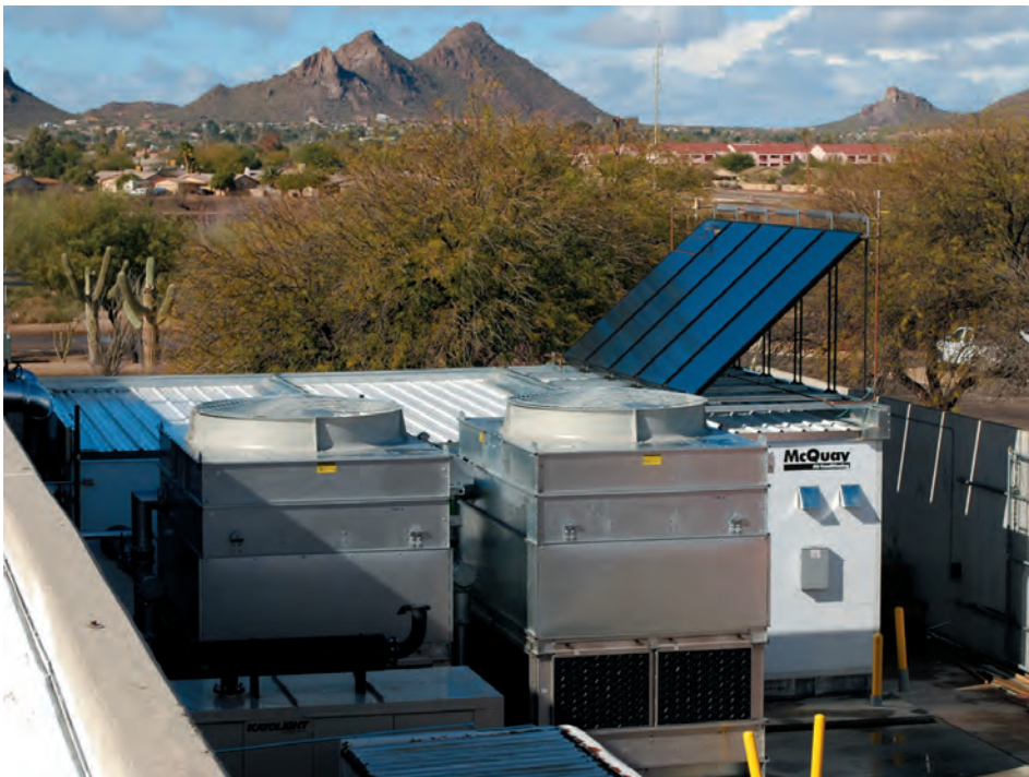
The Modular Central Plant at Pima Community College includes solar panels used to heat domestic water, further increasing energy costs savings.
