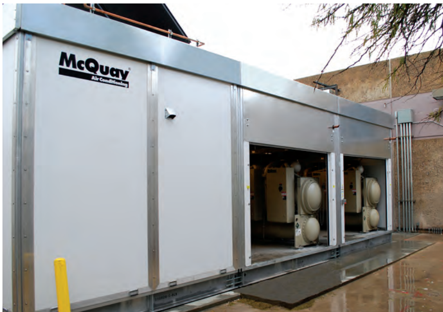
The Modular Central Plant includes two energy efficient, magnetic bearing compressor chillers that provide a big portion of the estimated 40% in mechanical utility cost savings.
