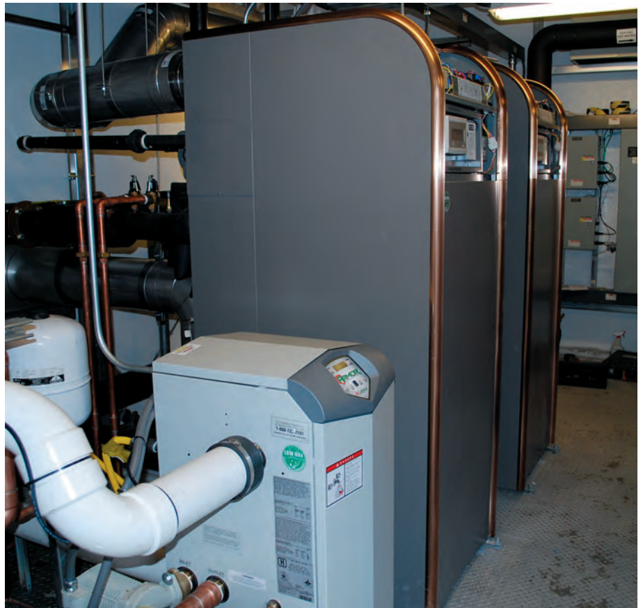
High efficiency sealed combustion natural gas boilers in the McQuay Modular Central Plant provide space heating to the Pueblo building on the Desert Vista campus.
