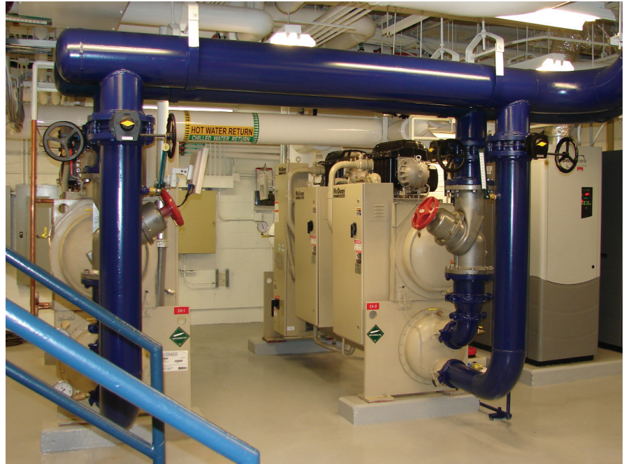
The chiller plant is located next to three classrooms in the lower level so the equipment had to be quiet. The McQuay WMC Chiller is the quietest chiller in its size range with sound pressure levels as low as 77 dBA per ARI Standard 575.
