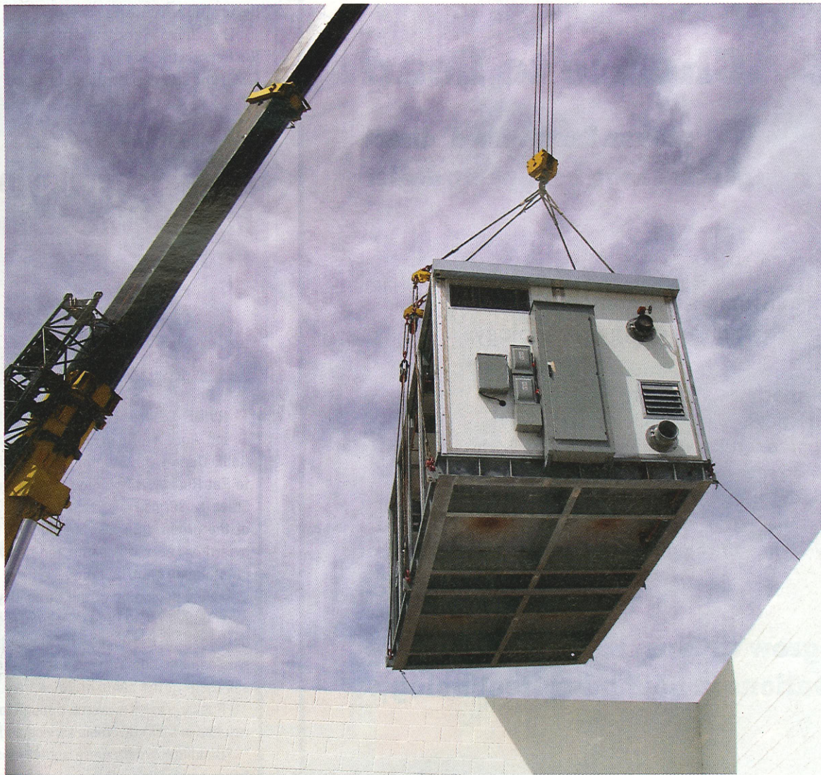
The chiller plant arrives at the jobsite as one pre-engineered and pre-assembled module ready for final assembly and hook-ups.
