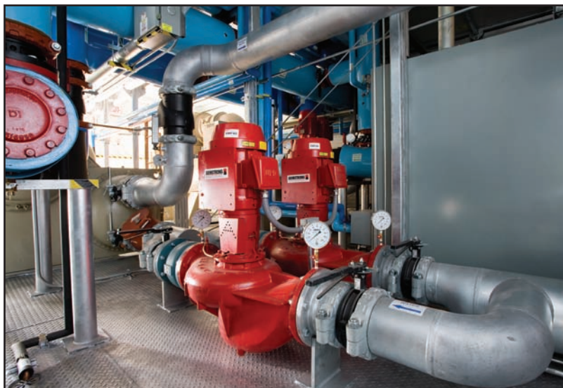
Phoenix NAP made extensive steps to ensure that the facility had fully redundant power and cooling systems.
