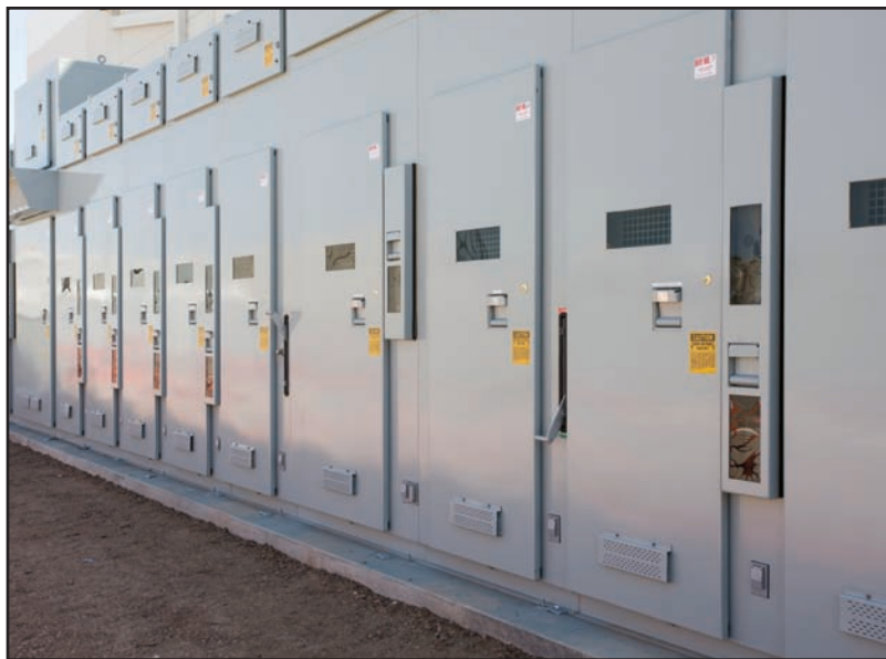
Siting the S&C switch gear and UPS systems in a secure yard freed valuable space inside the data center.
