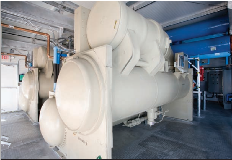
Phoenix NAP worked with McQuay International's Solutions Group to customize its MCPs to add more redundancies. The result was a product that McQuay states surpasses anything else they have available for that type of packaged chiller plant.
