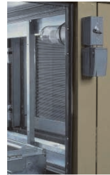
Lights and receptacles
