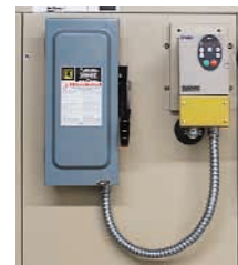
VFDs and disconnects
