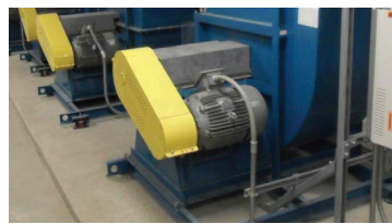
Teco 254T motor driving a RF4 AHU
